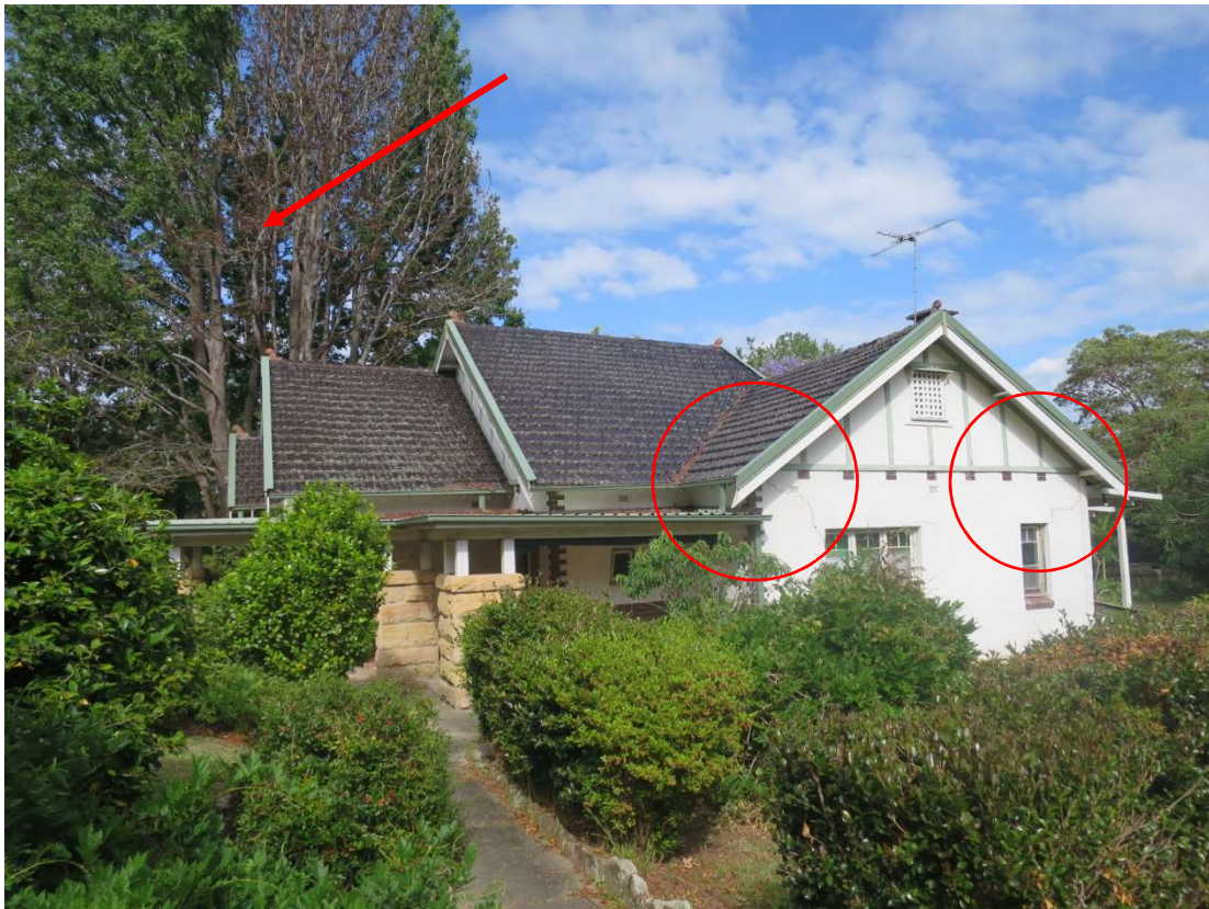
Figure 5 - View of the south eastern elevation showing the relationship between the tree on the adjacent site and the structural cracking on the diagonally opposite side of the building.
