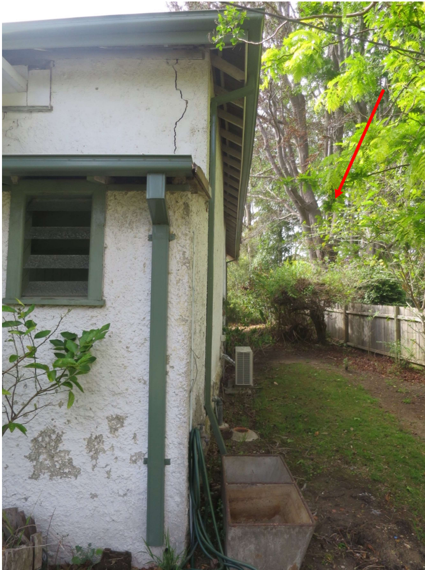
Figure 8 - Relationship of the adjacent tree and evidence of damage on the northern corner of the building.
