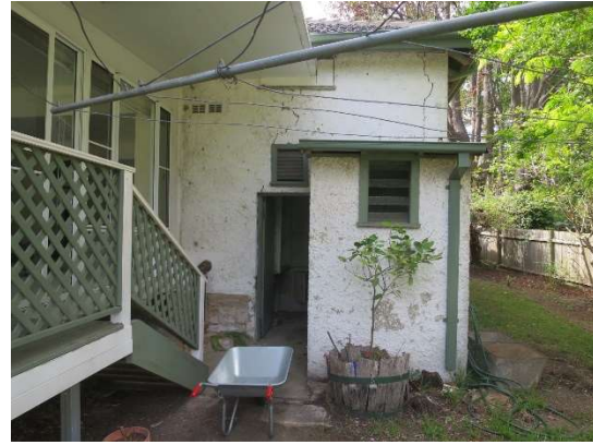
Figure 4 - View of a portion of the addition at the rear with structural cracking at the building corner.
