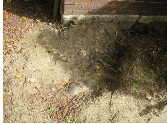
Figure 7 - Image showing the size of the root structure adjacent the building footings.
