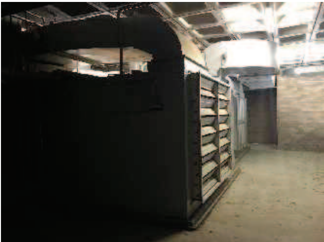
AUDITORIUM – PLANT AIR HANDLING UNITS AND DUCTWORK
