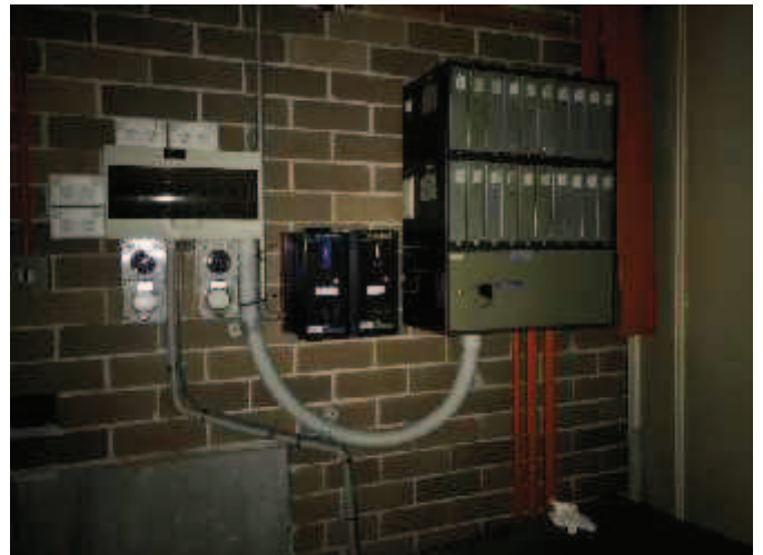
AUDITORIUM – PLANT CONTROLS
