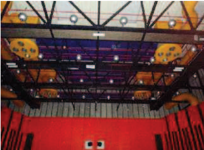
AUDITORIUM – CATWALKS LIGHTING ACOUSTICS, AIR CON DUCTS
