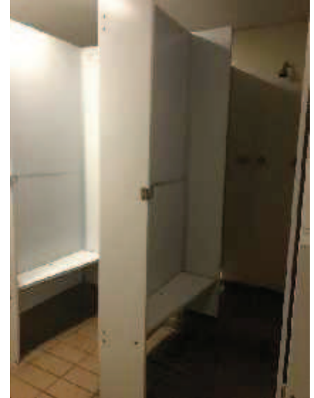
GYMNASIUM – SHOWER PARTITIONS
