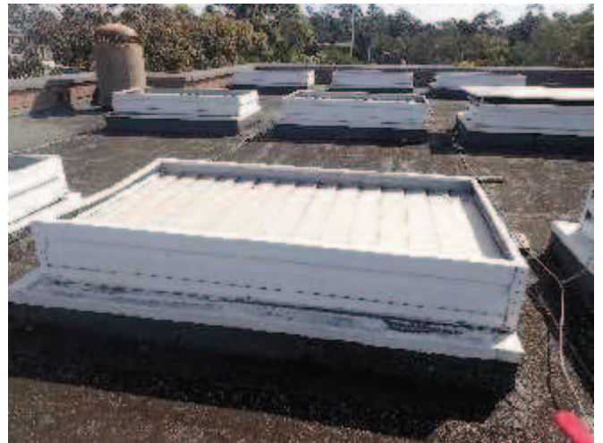
AUDITORIUM – ROOF MOUNTED SMOKE EXHAUST VENTS
